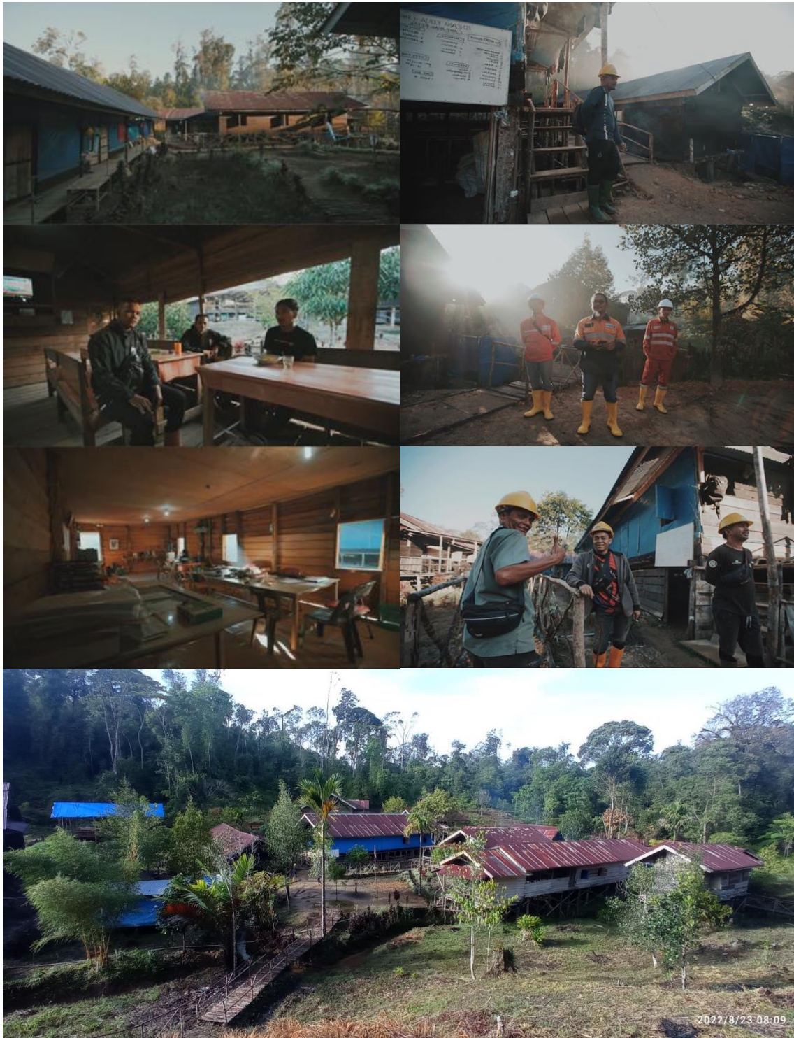
Figure 5: Images showing some of the upgrades to the Woyla Project base camp at Anak Perak.
